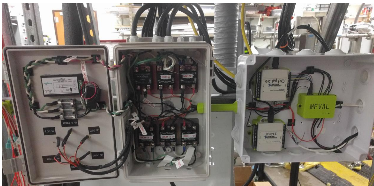
Figure 31: Left: Three-phase power box with fuses, indicator LED's, and six Solid-State Relays; Right: DAQs for interfacing with LabVIEW
