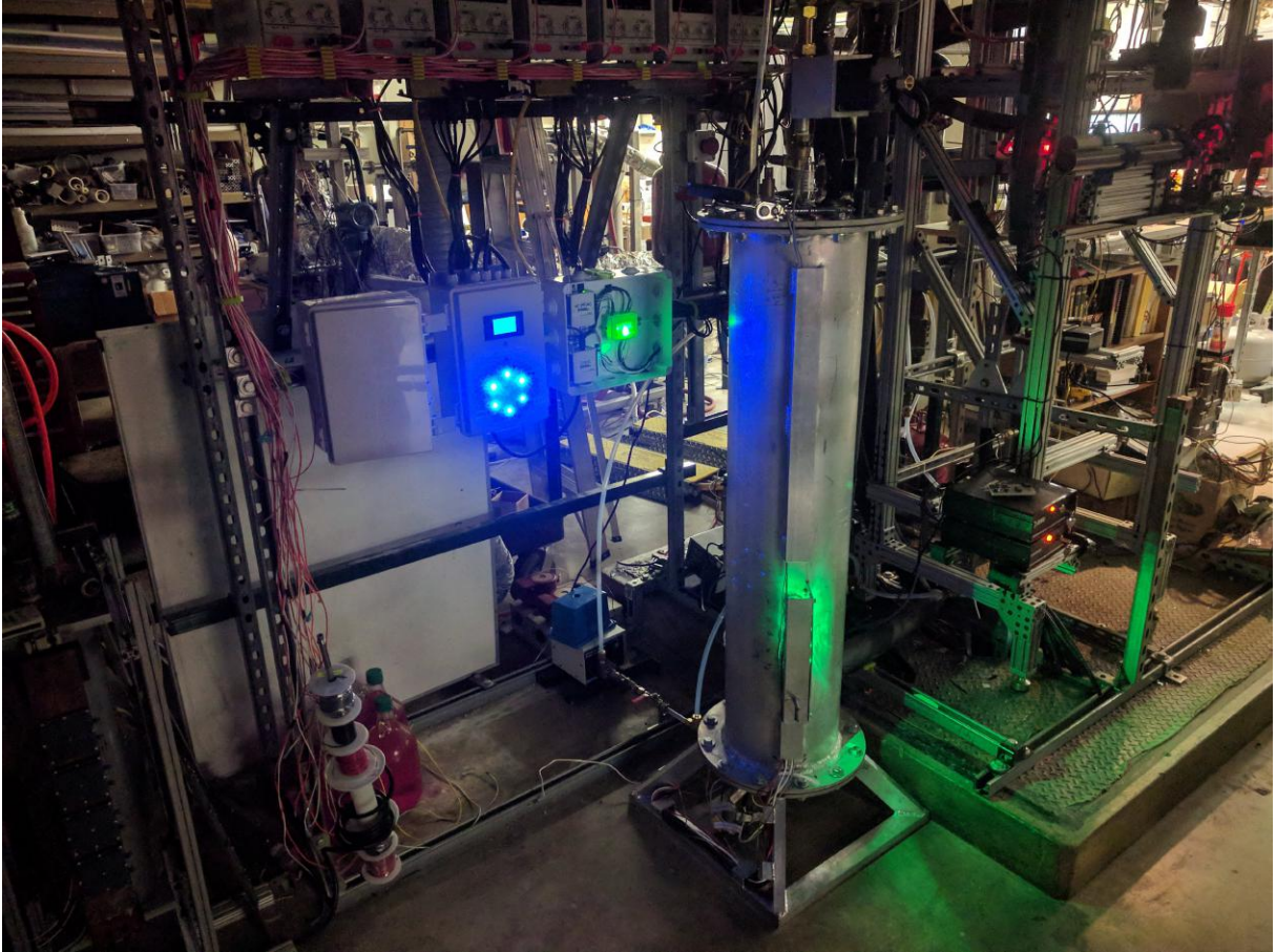
Figure 33: All six cartridge heaters and respective blue LEDs activated
